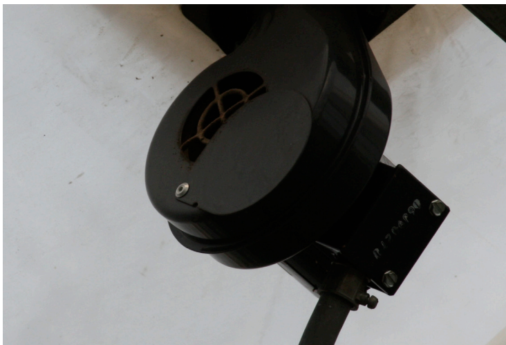
Figure 1. Inflation fans should use air from outside the greenhouse instead of from the inside to reduce the potential for humid air causing condensation between the two layers of poly.
